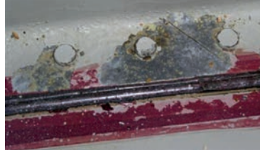
Figures 13 & 14 Missing/damaged protective treatments (Paint, primer, sealant, plating's, etc) will all allow ingress of fluids/corrosive products to cause corrosion damage, hence weakening the structure
