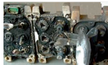
Figure 1 A short circuit caused by a contact pin burnt an A380 power distribution centre
