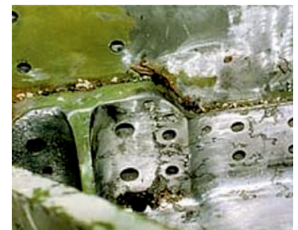
Figure 2 Example of pitting corrosion
