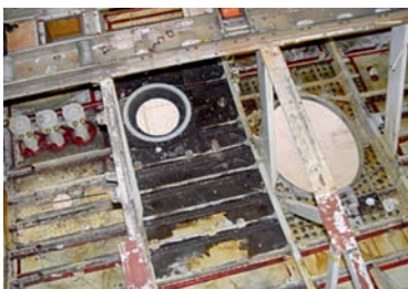
Figure 9 Corrosion through accumulation of dirt, debris and fluids in the bilge area
