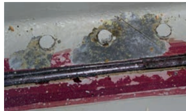
Figures 13 & 14 Missing/damaged protective treatments (Paint, primer, sealant, plating's, etc) will all allow ingress of fluids/corrosive products to cause corrosion damage, hence weakening the structure
